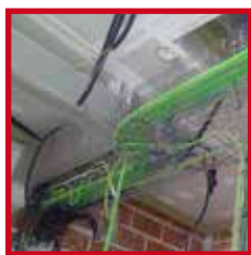
False floors and false ceilings
